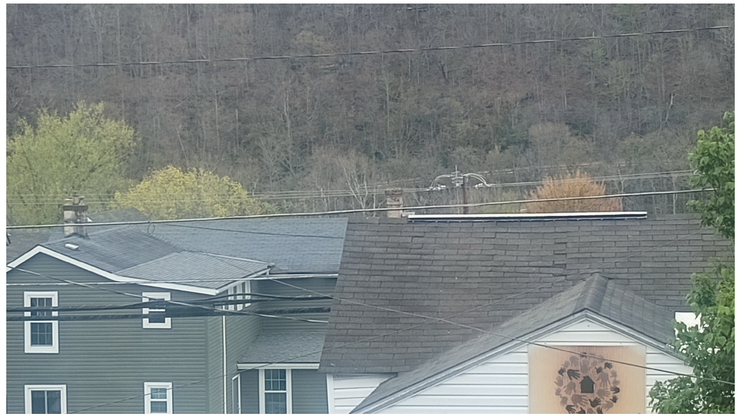
The roof of both the food pantry building and the child advocacy center
